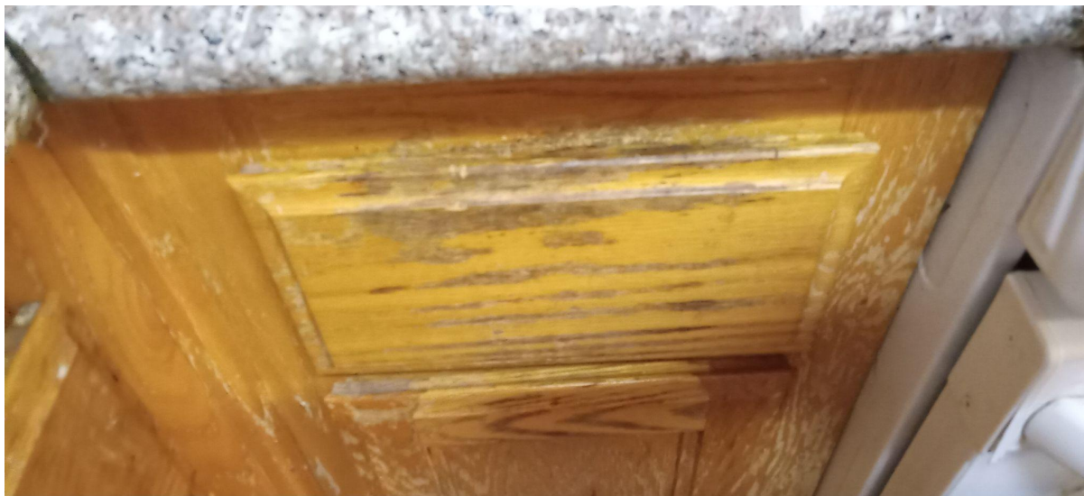
2 Tenant #1 - Mold in the Kitchen
