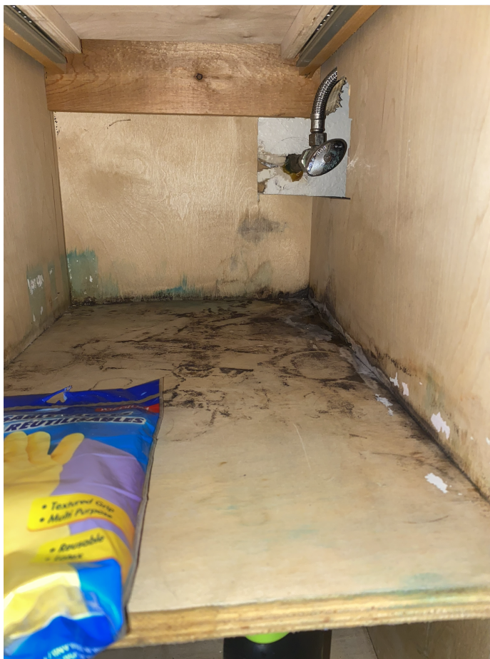
4 Tenant #2 - Mold underneath the kitchen sink due to leaks
